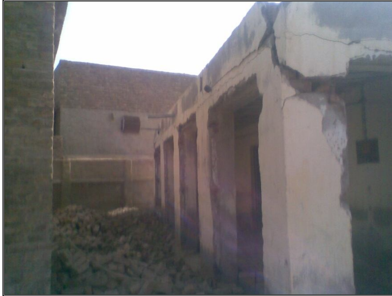
Deteriorating Condition of Govt Girls Primary School Mir Muhalla Khadro, District Sanghar.
